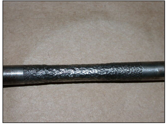
Corroded Attach Bolt
