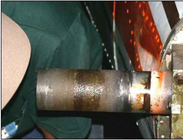
Corroded Torque Tube (PA-24)
